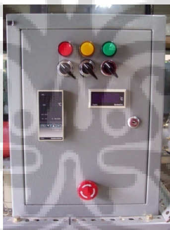
Gambar III.11 Panel Sistem Listrik
