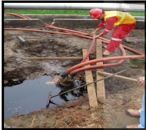
Gambar 6.14 Insiden kebocoran bottom plate
