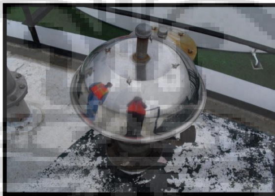
Gambar 5.7 Pressure Vacuum Vent
