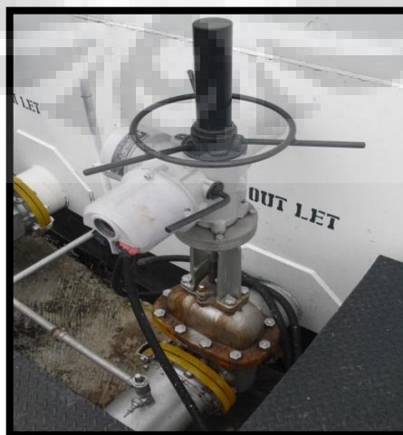
Gambar 5.2 MOV ( Motor Operated Valve )
