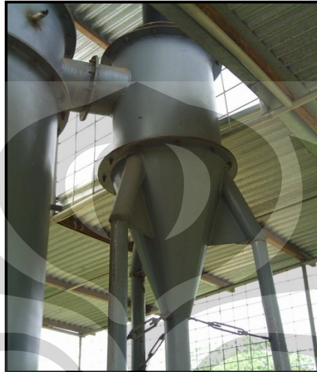
Gambar 2.13 Cyclone Separator Fluidized Bed Combustor UI
