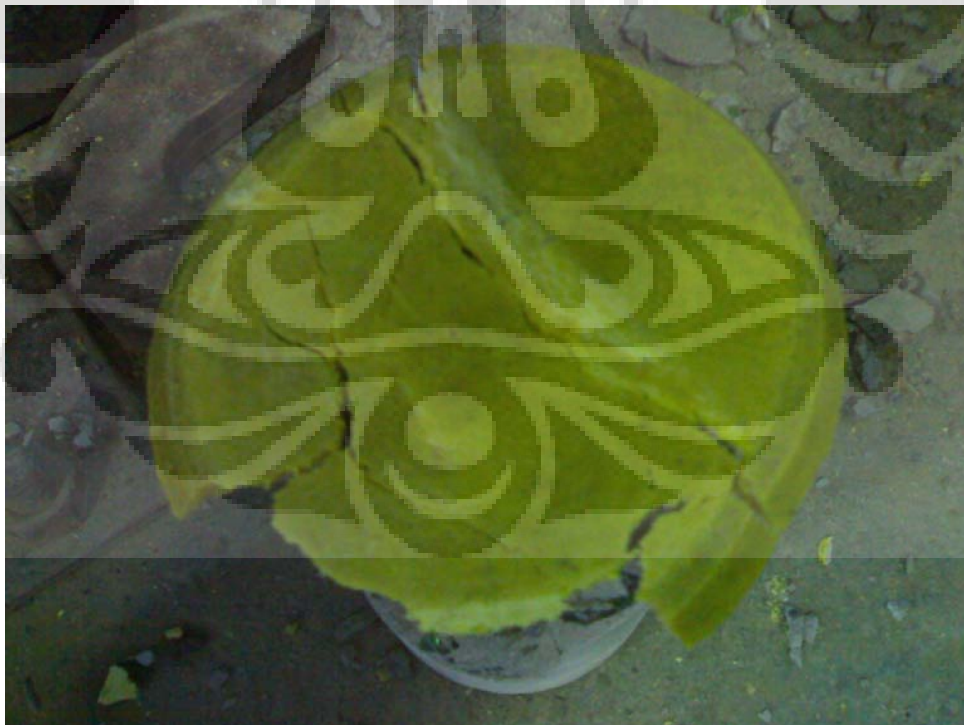
Detail keruntuhan capping miring
