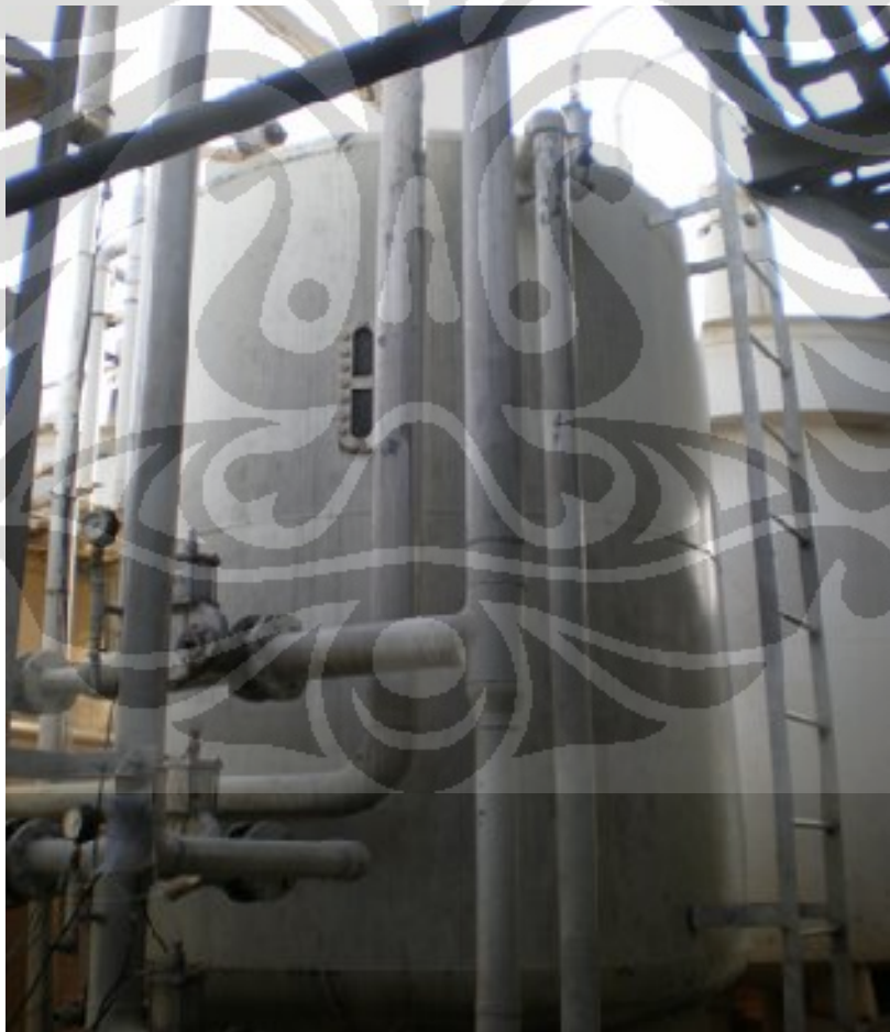
Gambar 4.7. Unit Filtrasi ( sand filter )
