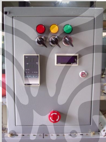
Gambar III.10 Panel Sistem Listrik
