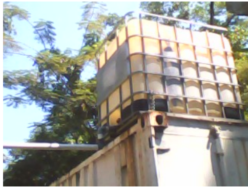
Gambar 3.2.3 Reservoir Air Utama
