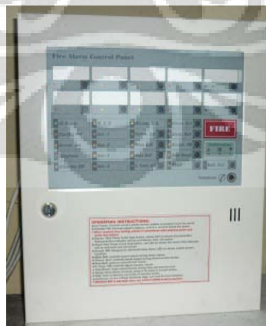
Gambar 2.6 Panel alarm kebakaran
