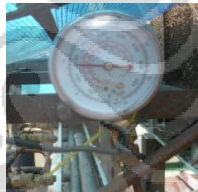
Gambar 3.22 Pressure Gauge outlet kondenser
