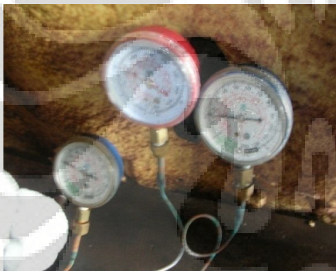
Gambar 3.21 Pressure Gauge inletTXV, outlet TXV, dan outlet evaporator
