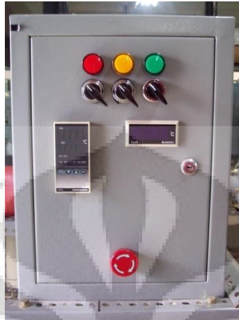
Gambar III.11 Panel Sistem Listrik
