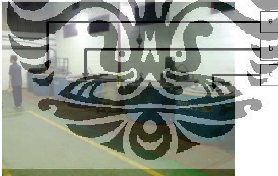
Gambar 4.3. (a) Tungku preheating. (b) Tungku austenisasi. (c) Tungku austempering.
