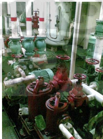
Gambar 3-6. Gambar Fo. Transfer Pump
