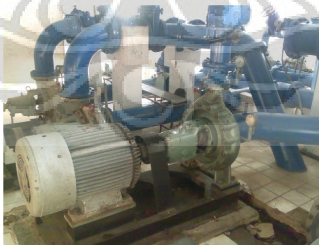
Gambar 4.4 Pompa Distribusi Cabang 3
