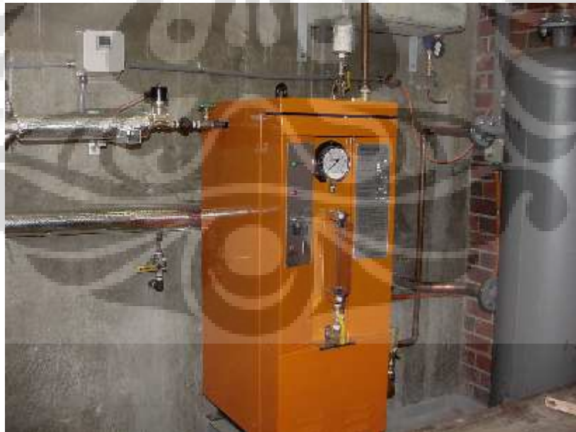
Figure 3.13: Steam Boiler and Controls
