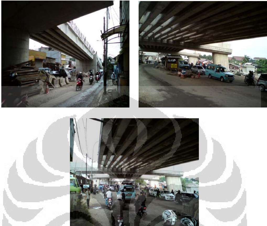
Gambar 1.2 Kondisi Jembatan Flyover Kalibata (8 November 2010)
