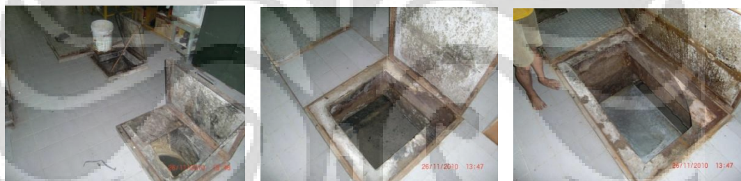
Gambar 4.8 Grease trap Restoran Nelayan
