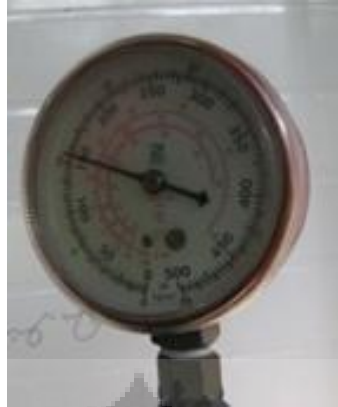
Gambar 3. 8 Pressure gauge jenis hi pressure
