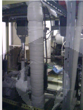
Gambar 3-5 Cascade heat exchanger
