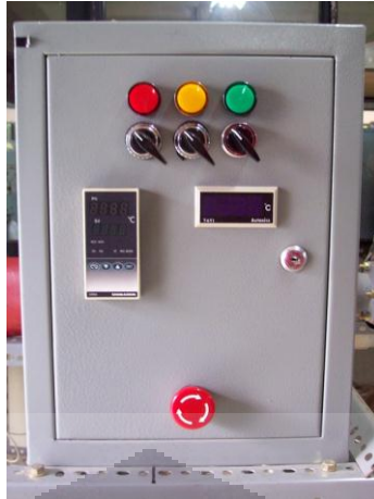
Gambar III.13 Panel Sistem Listrik
