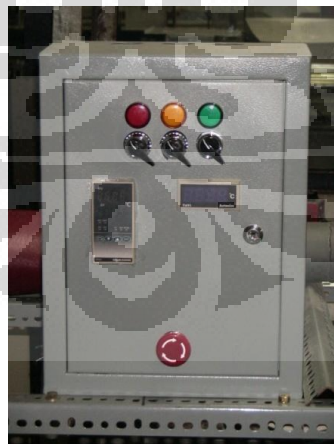
Gambar III.11 Panel Sistem Listrik
