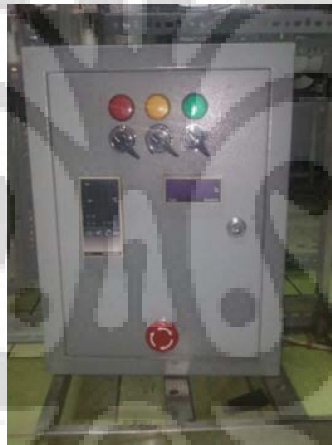
Gambar III.12 Panel Sistem Listrik
