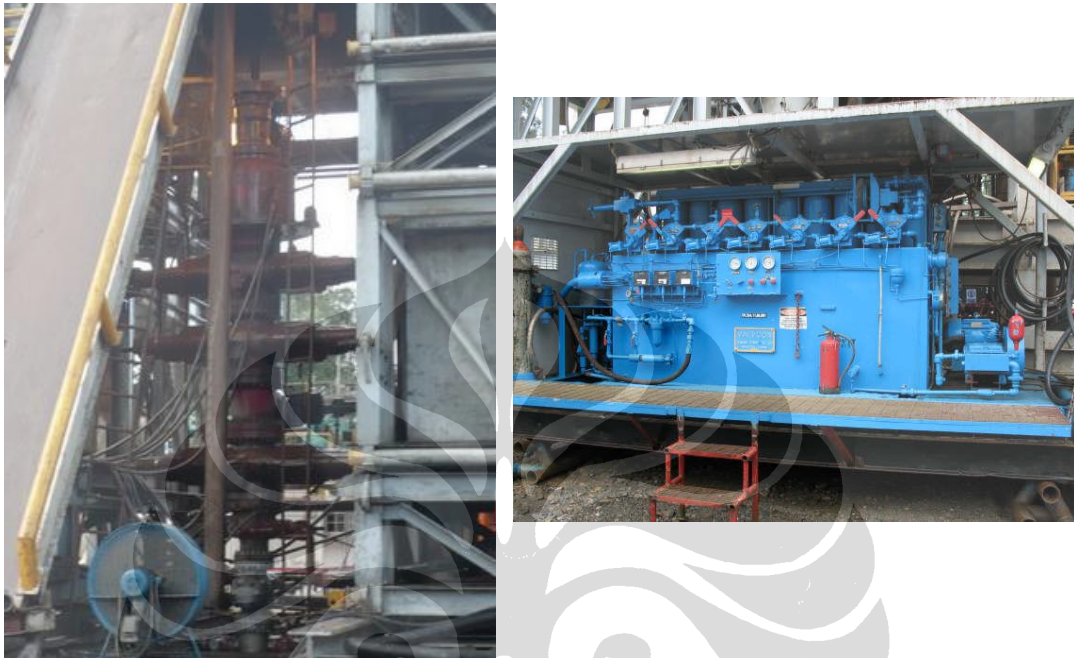
Gambar 6.5. BOP ( Blowout Preventing System ) & Koomey
