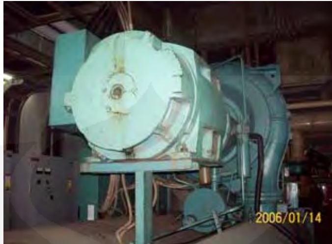
Gambar 3.1 Motor Chiller YORK
