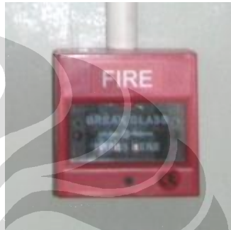
Gambar 6.6 Titik Panggil Manual ( Manual Station ) Di PT. X Jakarta
