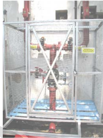
Gambar 6.11 Main Valve Sprinkler System
