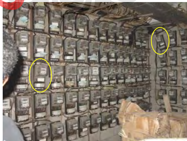
(a) kWh Meter Miring
