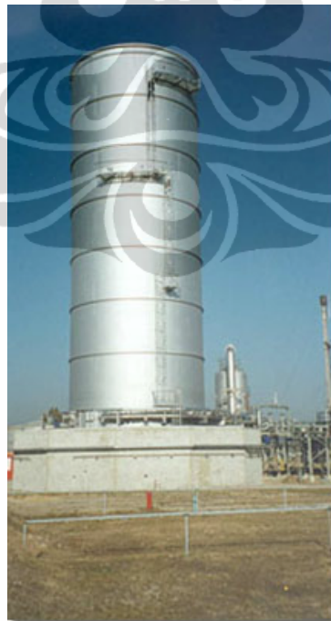
Gambar 2.1. Stack Enclosed Ground Flare [6]
