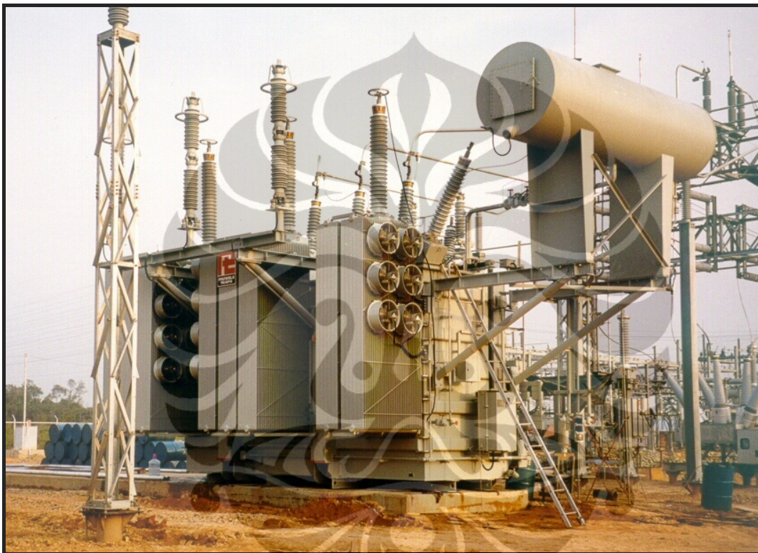
Gambar 3.1 Pauwels trafo 132/66 kV – 100MVA
