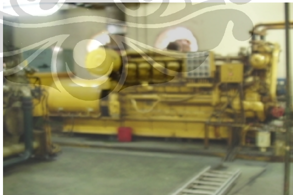
Gambar 2.4 Generator Diesel Gedung RS Dharmais
