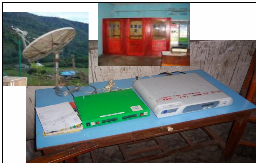
Gambar 3.2. Komponen Teknologi Very Small Aperture Terminal (VSAT) [8]
