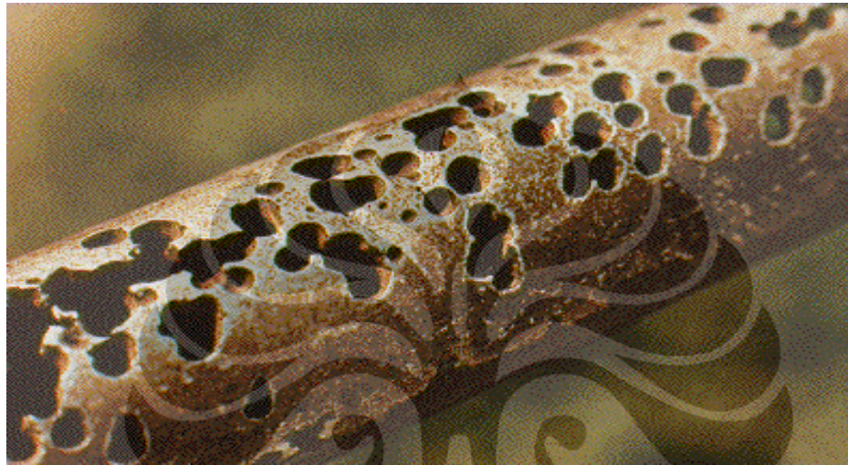
Gambar 1.1. Pitting Corrosion Pipa Boiler & Cooling Water [22]
