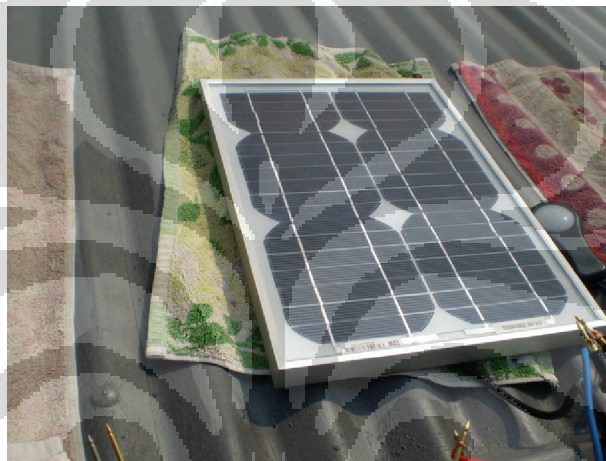
Gambar.4.27. Charging Solar Cell
