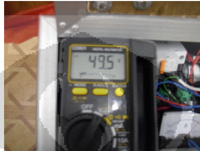
Gambar.4.29. Sistem Pengukuran Charging Generator
