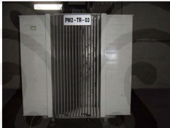
Gambar Trafo Distribusi PM2-TR-03, 6.3 KV/380 V
