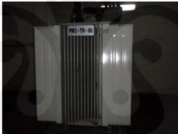
Gambar Trafo Distribusi PM2-TR-06, 6.3 KV/460 V
