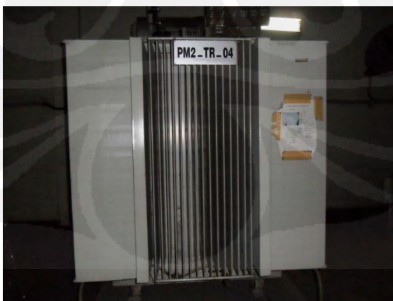
Gambar Trafo Distribusi PM2-TR-04, 6.3 KV/380 V
