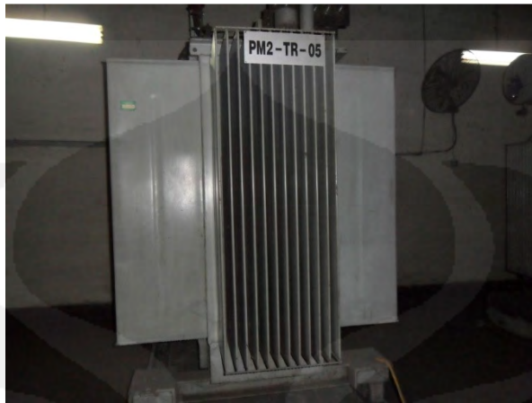
Gambar Trafo Distribusi PM2-TR-05, 6.3 KV/380 V
