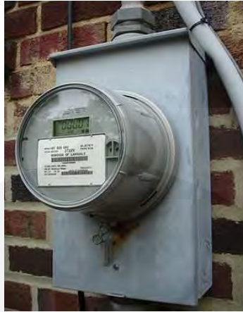
Gambar 2.1. Automatic Meter Reading (AMR) [1]
