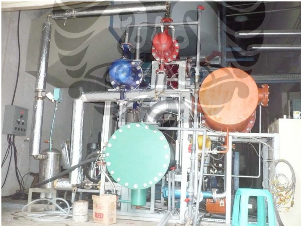
Gambar 4.1. Mesin Absorption Chiller
