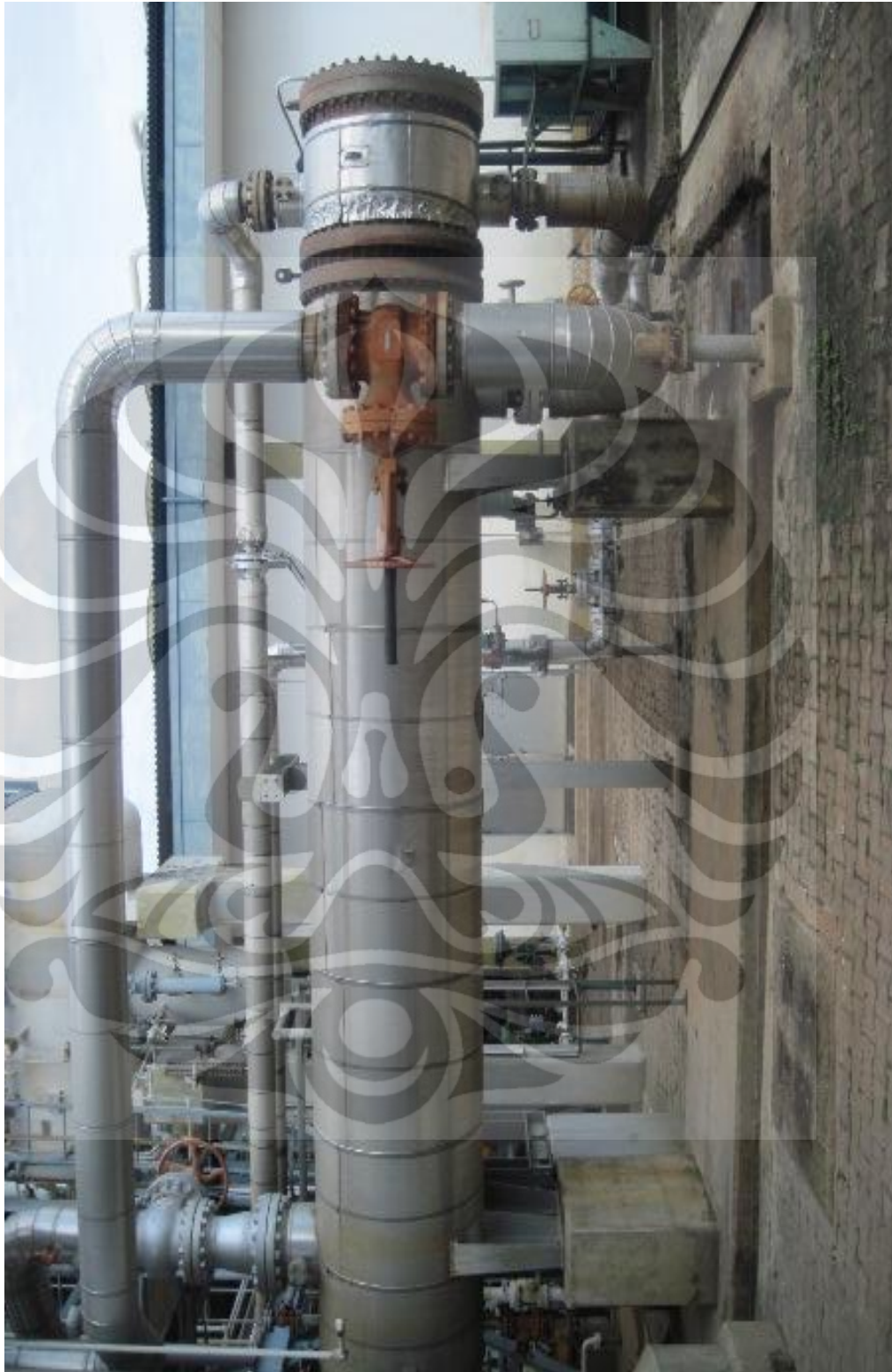
Gambar 4.2. Instalasi Unit HE – 7
