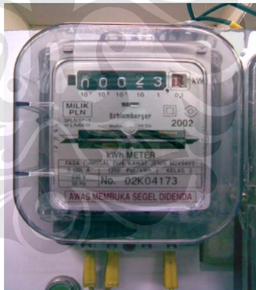
Gambar 3.2 KWh-meter satu fasa Schlumberger
