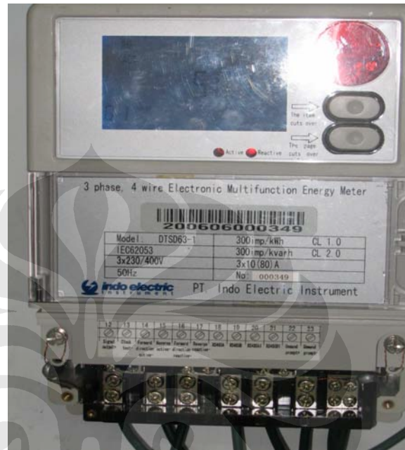
Gambar 3.5 KWh-meter tiga fasa PT. Indo Electric instrument
