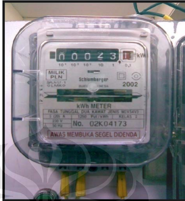
Gambar 3.2 KWh-meter satu fasa merk Schlumberger
