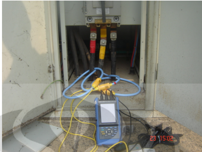
Gambar 3.12 Panel MCB chiller
