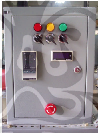
Gambar III.12 Panel Sistem Listrik
