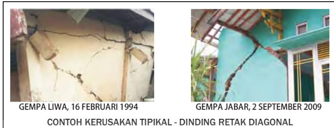
Gambar 1. 4. Dinding Bata Retak Diagonal Akibat Beban Lateral (Sumber: Boen, Teddy and associates, 2010)
