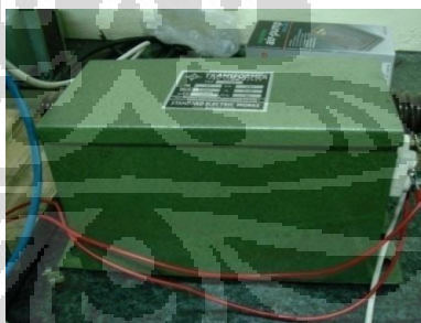
Gambar 3. 8. Neon Sign Transformer
