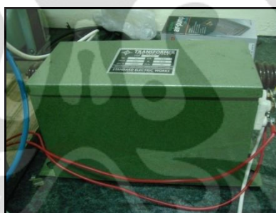
Gambar 3. 7. Neon Sign Transformer
