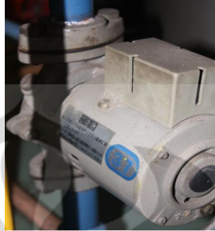
Gambar 3.17. Feed Water Pump
