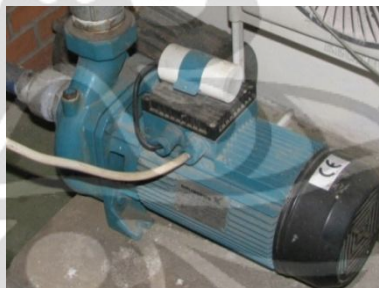
Gambar 3.18. Circulating Water Pump
