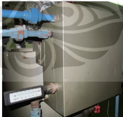
Gambar 3.10. Feed Water Tank
