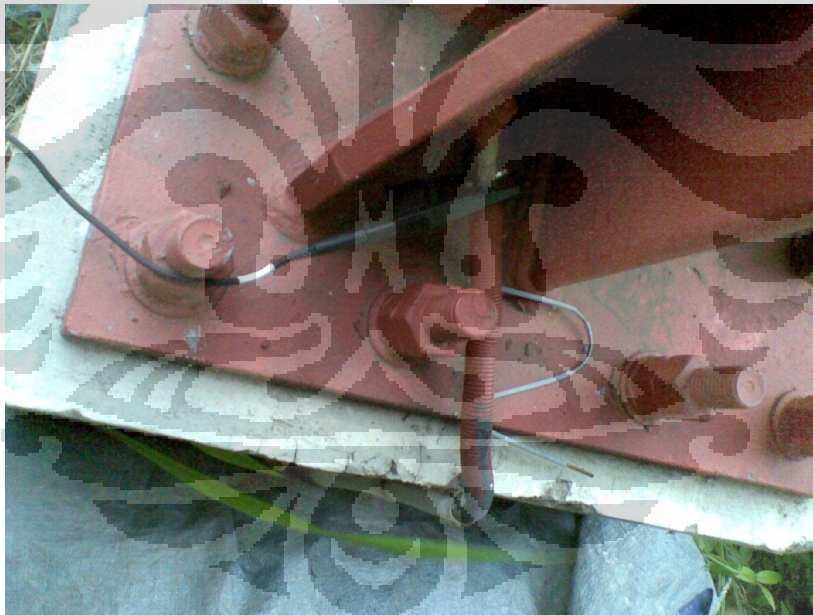
Posisi Grounding System
