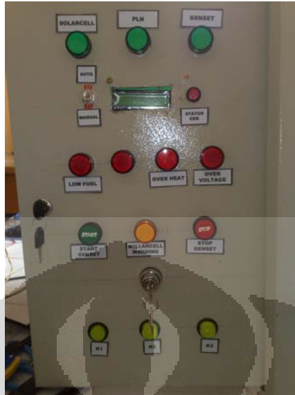
Gambar 3.20. Box Panel Sistem Kontrol
