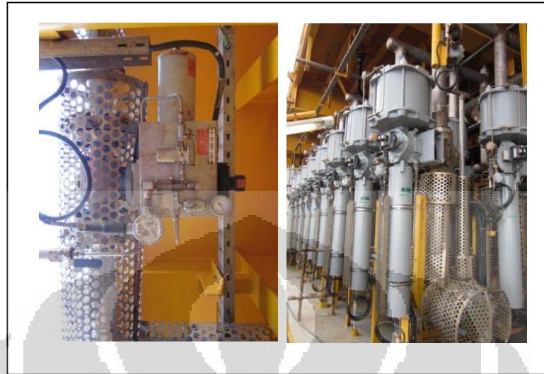
Gambar 4.7. Fasilitas Emergency Shutdown dan Blowdown Valve
