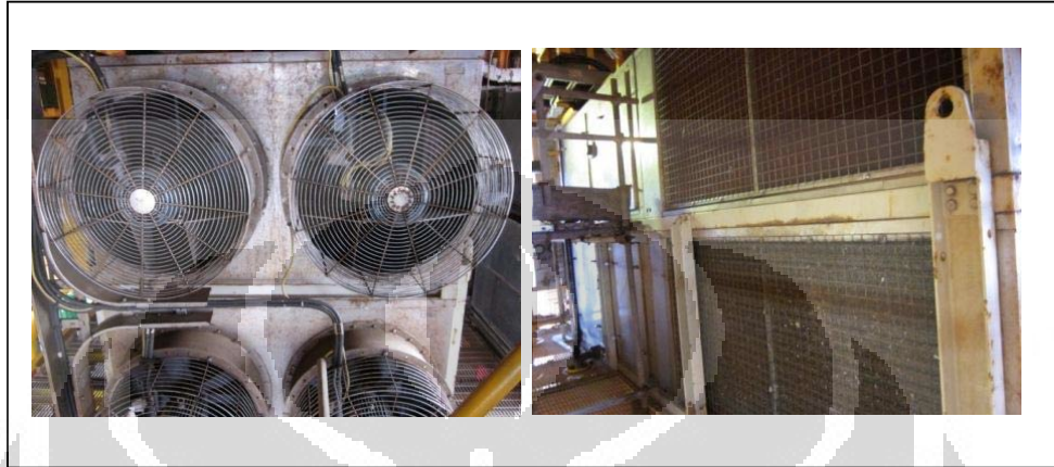
Gambar 4.9. Fasilitas HVAC ( Heating Ventilating Air Conditioning )
