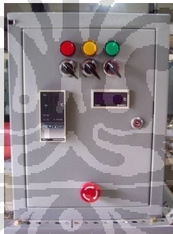
Gambar IIL11 Panel Sistem Listrik
