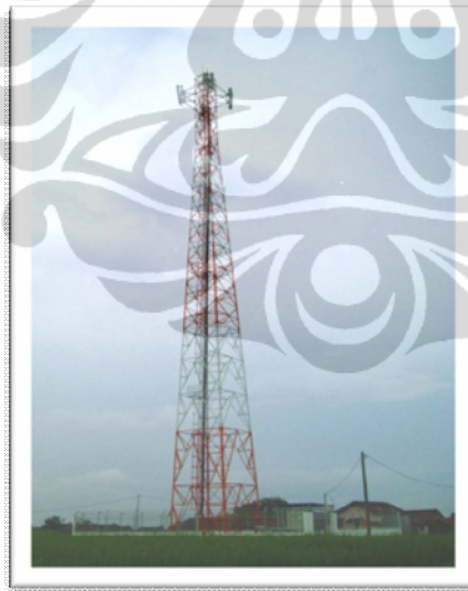
Gambar 2.2 Tower SST Green Field
