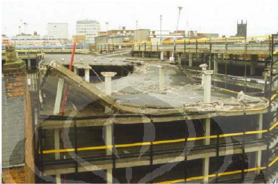
Gambar 1.2 Fenomena Kegagalan Punching Shear
