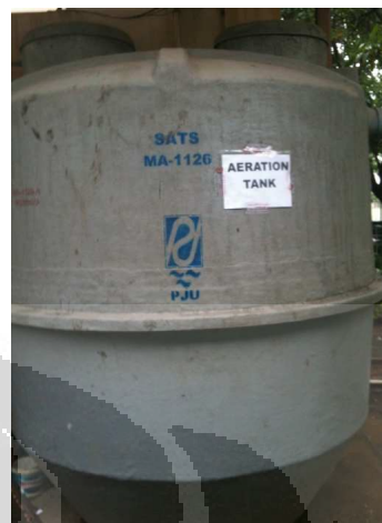
Gambar aeration tank
